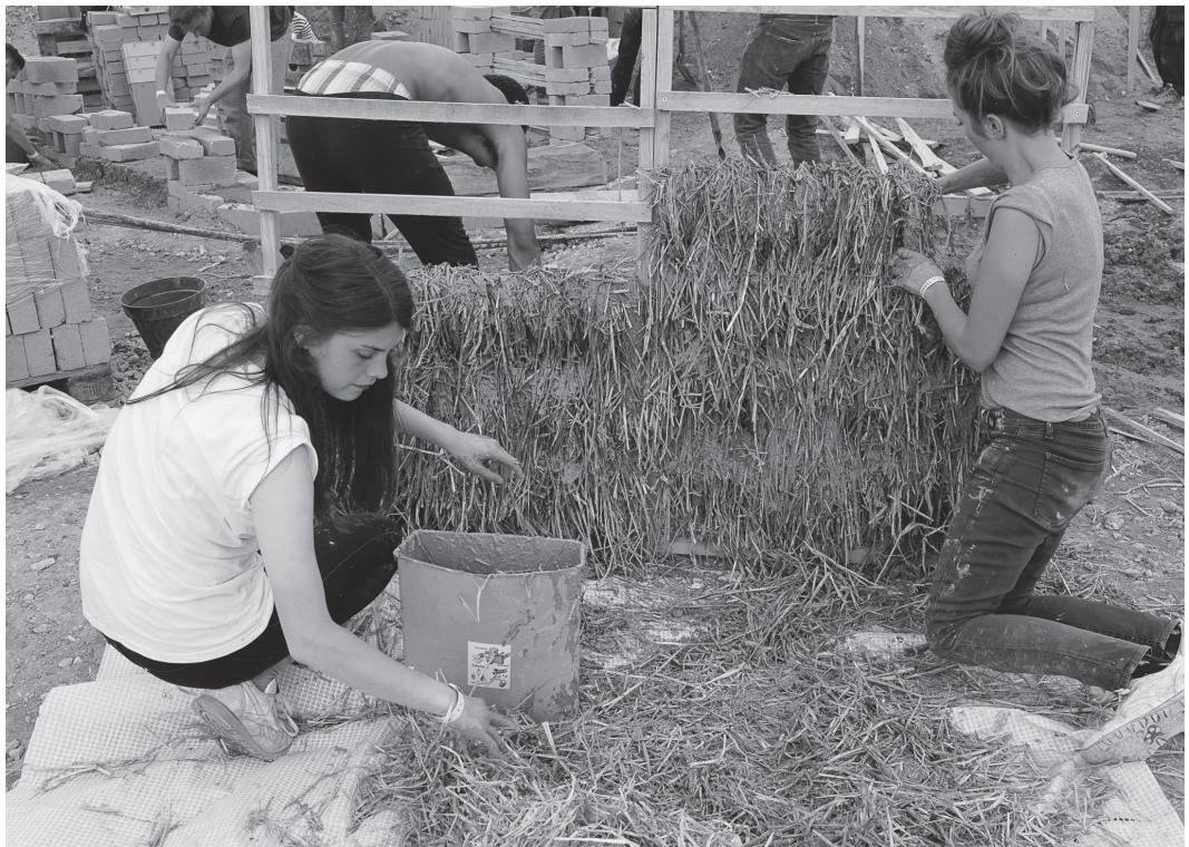
CATTAIL CATTAILS ARE MADE WITH THE MEANS OF THE EDGE AND ALLOW TO LIGHTEN THE STRUCTURES OF THE SHELTERS. PHOTO BY SANDRINE MARC
