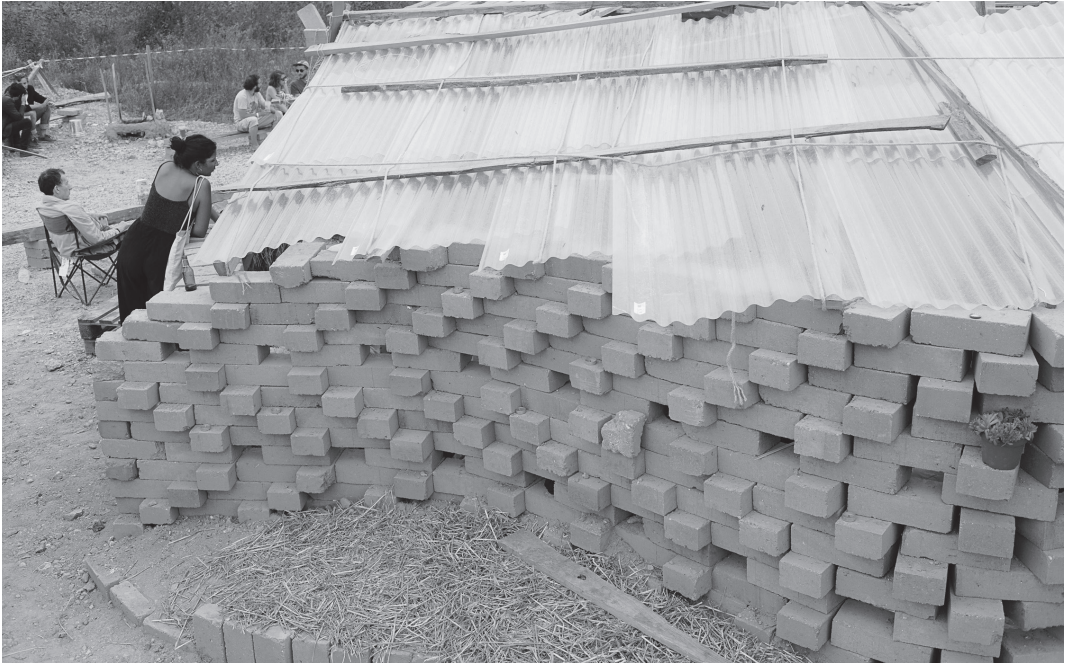
FESTIVAL-GOERS REDOUBLE THEIR IMAGINATION TO IMPLEMENT SOLID STRUCTURAL WALLS IN CEB WITHOUT MORTARS. THE RESULT IS ORIGINAL FITTINGS AND MOUCHARABIEH (CLAUSTRA) AND CURVED ORGANIC WALLS. PHOTO BY ALEXIS LECLERCQ
